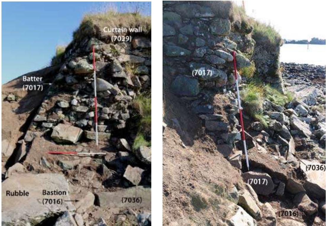
Figure 13 Left: Annotated structural components at the northwest corner of the outer courtyard showing the relationships between bastion (7016), earlier curtain wall face (7036), later curtain wall (7029) and batter (7017); Right: view of batter (7017) and surviving bottom course of curtain wall (7036) in relation to the better surviving face of the curtain wall on the same line in the background demonstrating the volume of masonry lost to erosion.
