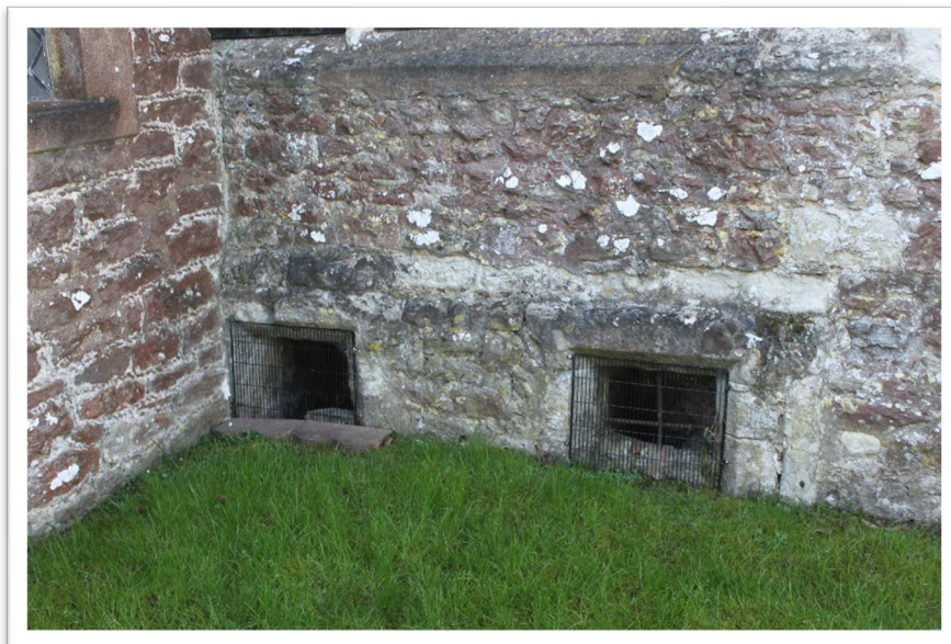
(Fig 34: East-facing north aisle wall which provided access for video cameras to film the crypt)
