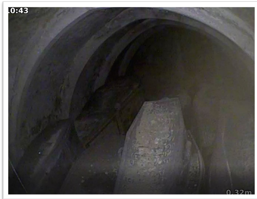
(Fig 33: Looking west through crypt air grate at coffins and vaulted ceiling, source: Mr Francois Gordon)
