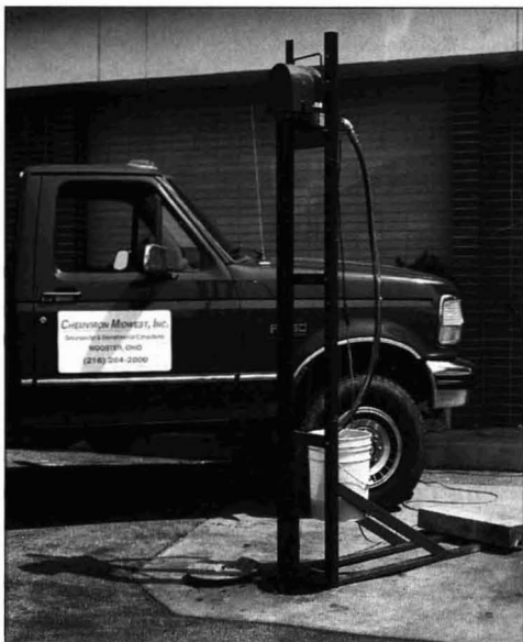
An Abanaki PetroExtractor and mounting stand being used for oil recovery at an Ohio service station site.
