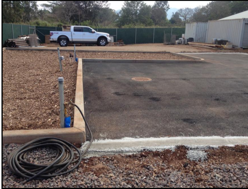
The West Base wash rack consists of a paved surface for washing, which drains into a bioretention area. The bioretention area currently is mulched and awaiting planting.
