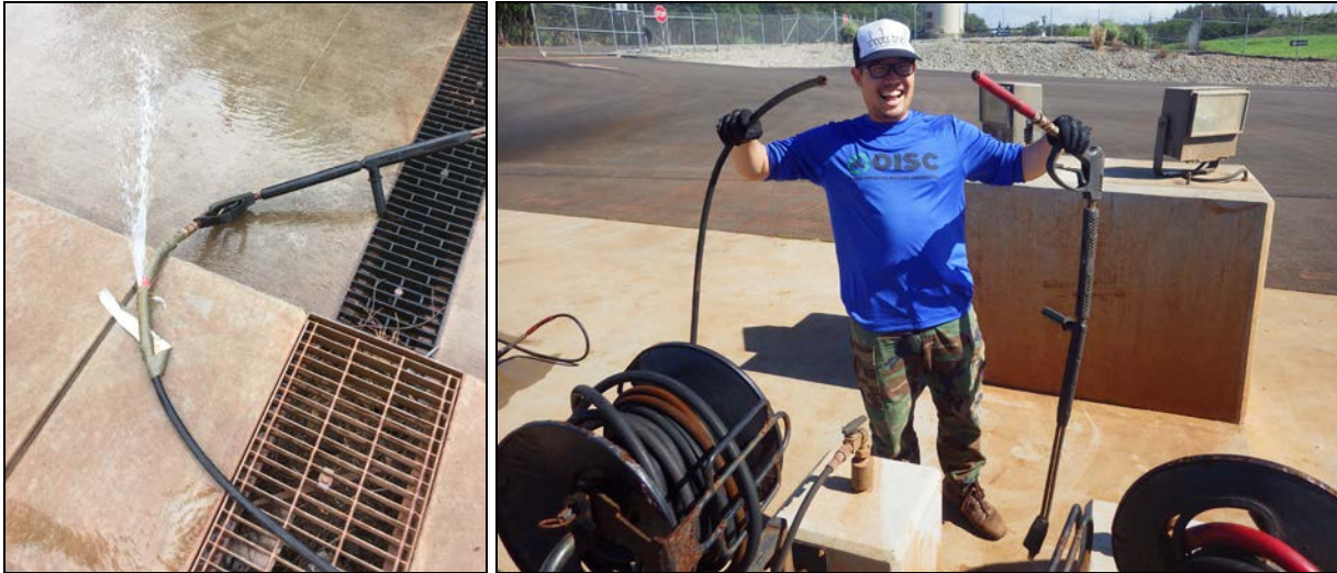
Figure 10. Leaking and broken pressure hoses.
