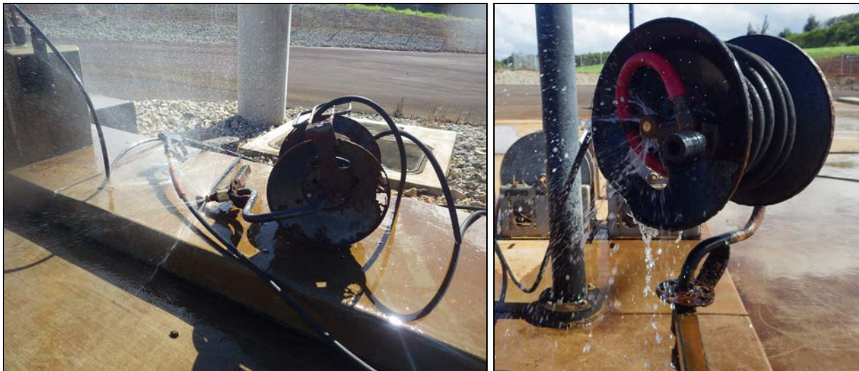
Figure 9. Left: this hose reel is detached from its mount and now sits on the ground, the reel is rusted through, and water leaks from all connecting points. Right: while still on its mount, this hose reel leaks prolifically.
