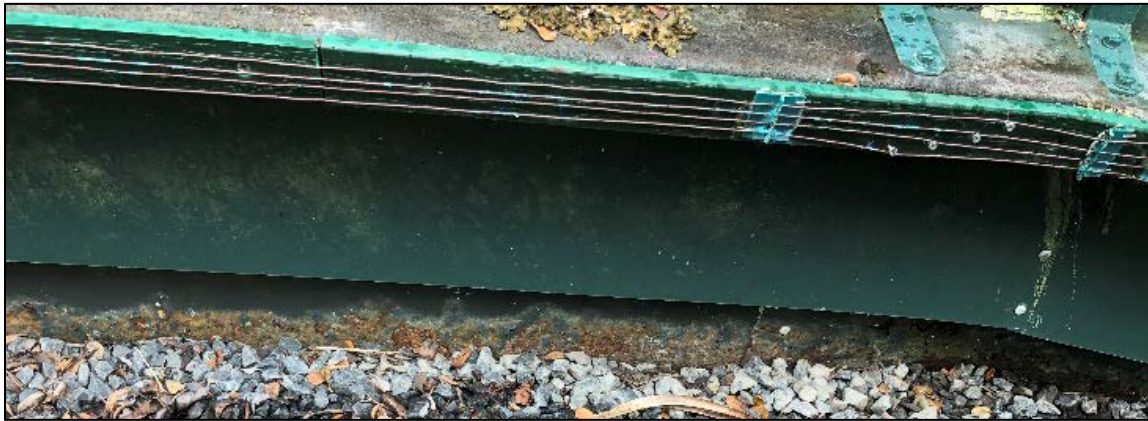
Figure 28. Corrosion at base of Palikea South enclosure wall
