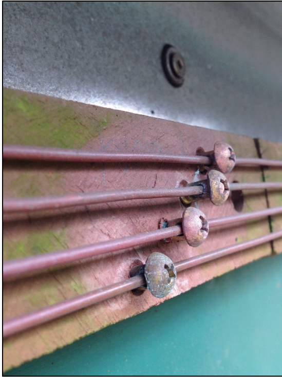
Figure 25. Copper wires held in place by stringing through holes drilled in brass screws.
