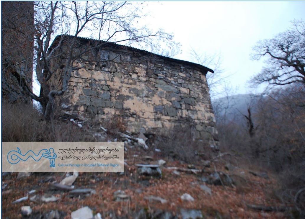
Figure A.1.18: Tsinkibe Fortress Complex, St. Barbare church in 2009 © Blue Shield Georgia
