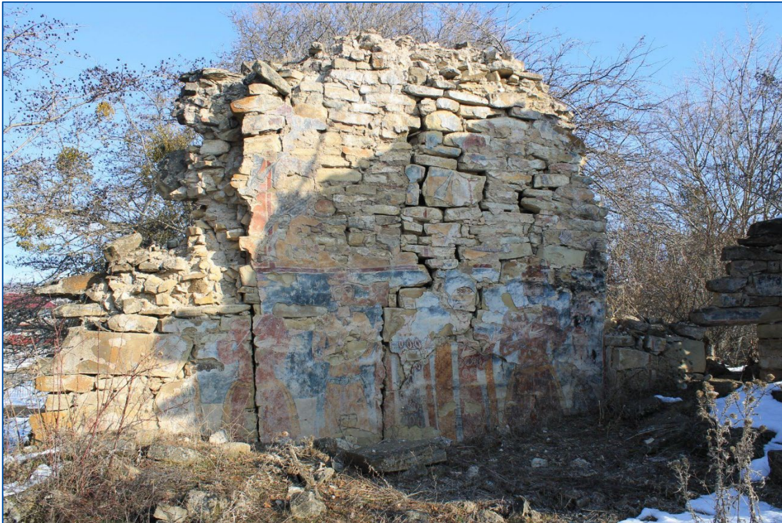
Figure A1.77: Vakhtana Church of the Virgin, the Northern wall (2014) © Didi Liakhvi Valley Museum-Reserve
