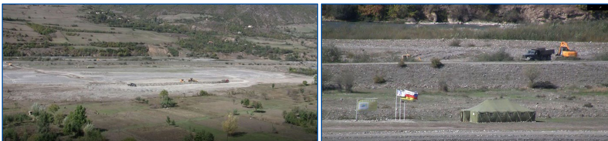
Figure A1.32, A1,33: Historic Orchards of the palace being bulldozed (2010) © Didi Liakhvi Valley Museum-Reserve
