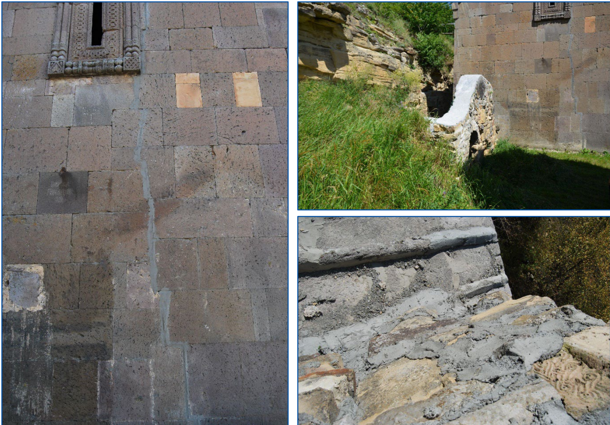
Figures A1.56a,b,c: Use of cement in the reconstruction and repair work at Tiri Monastery, 2016. ©Blue Shield Georgia.
