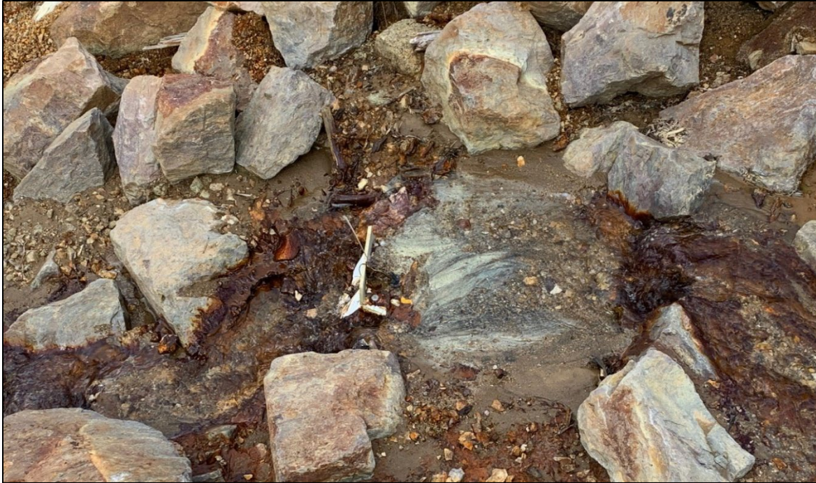
Figure 4. Upper Bullion flume filled with sediment after summer rain event.
