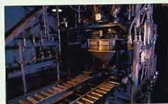
Engineering, procurement and construction management services are being provided by Fluor Daniel's Government Sector to TRW for a new auto air bag propellant and assembly plant in Mesa, Arizona.
