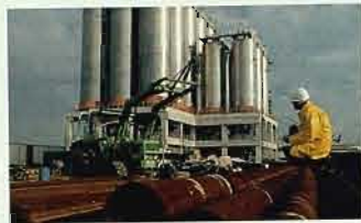
Fluor Daniel's Hydrocarbon Sector provided a full spectrum of services from design through construction management and startup assistance for a Shell grass roots polypropylene plant near Cologne, Germany.
