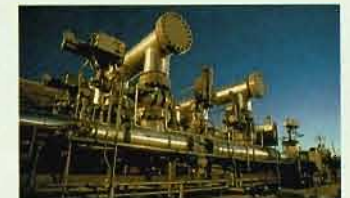
Engineering and construction management was provided to the DOE by Fluor Daniel's Government Sector for a 13-mile pipeline and meter station connecting to the West Hackberry Strategic Petroleum Reserve (SPR). The first SPR sale passed through this system in October.
