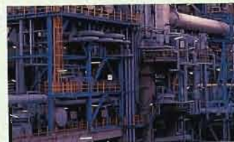
Engineering and procurement services for a high vacuum unit at Veba Oel's refinery complex in Gelsenkirchen, Germany were performed by Fluor Daniel's Hydrocarbon Sector.
