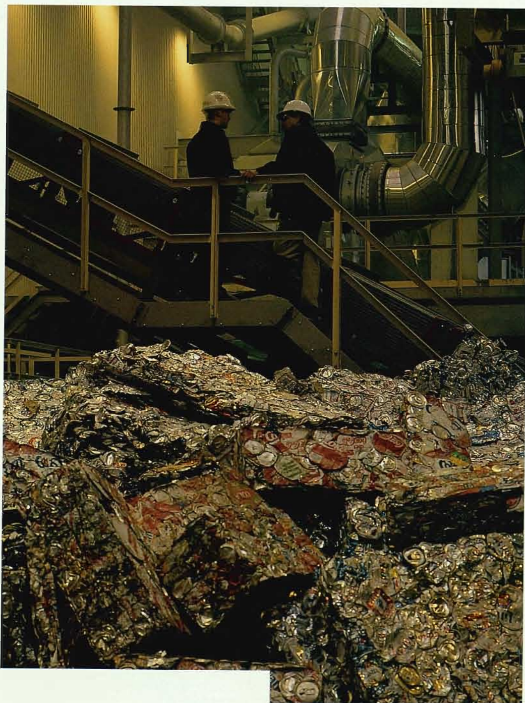
In a global expansion of Fluor Daniel's nearly four-year alliance with Alcan, the Industrial Sector provided total responsibility services to British Alcan Aluminum to construct a used beverage can recycling plant in the U.K. Modeled after a sister facility also built by Fluor Daniel in Berea, Kentucky, the plant is the first in the European Economic Community fully dedicated to aluminum can recycling and is capable of processing 9 million cans per day.
