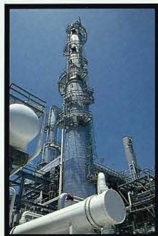
Recent project assignments at the Valero Refinery in Corpus Christi, Texas include the addition of an MTBE plant
