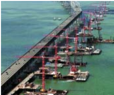
Potain tower cranes are the leading brand in a growing global market. A range of 77 models, including these MD 560's, are ideal for a wide range of applications including bridge, infrastructure, and commercial construction.
