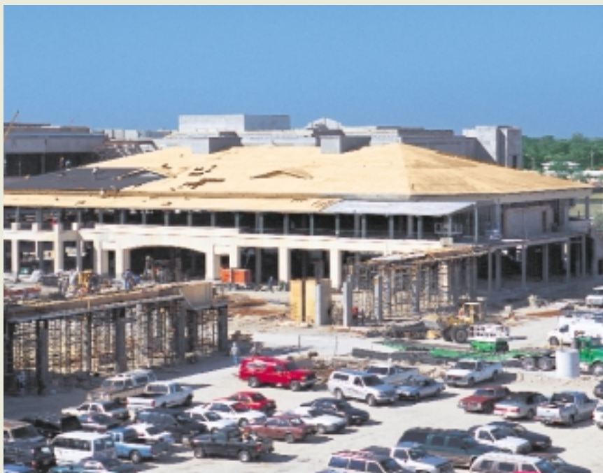
Construction is on schedule for the September 27, 2002 opening of the Village of Merrick Park.
