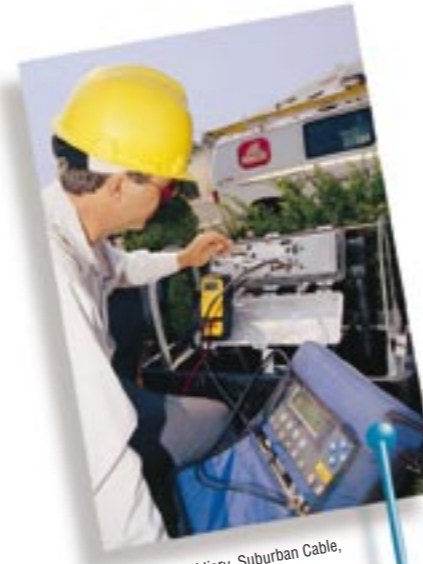
Lenfest subsidiary, Suburban Cable, is upgrading networks to offer advanced services to customers
