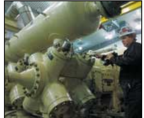
▲ Mechanic Gene Turner uses a gas leak detector as he readies some of the systems at the Lodi natural gas storage facility in California.
