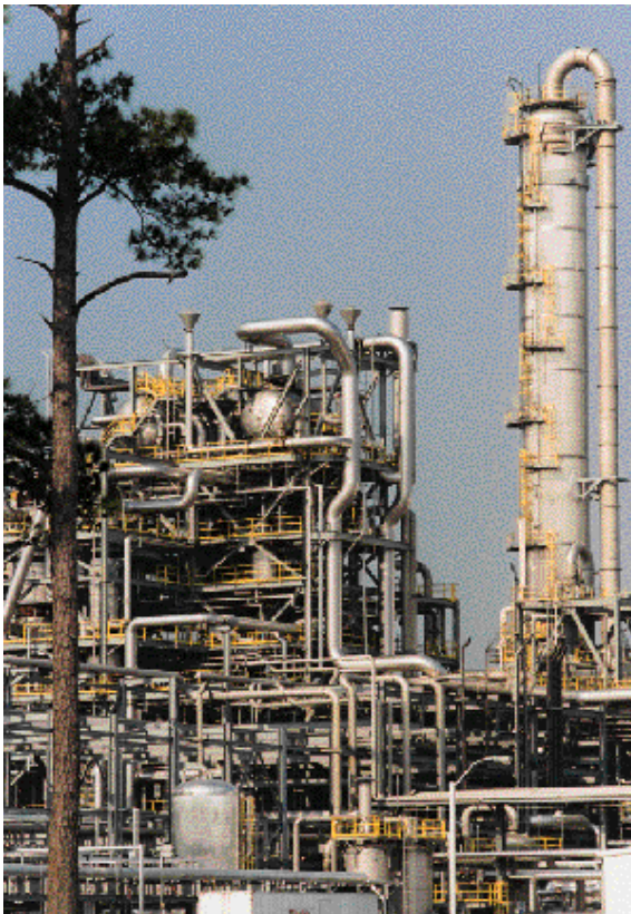
Cooper River PTA plant - U.S.A
