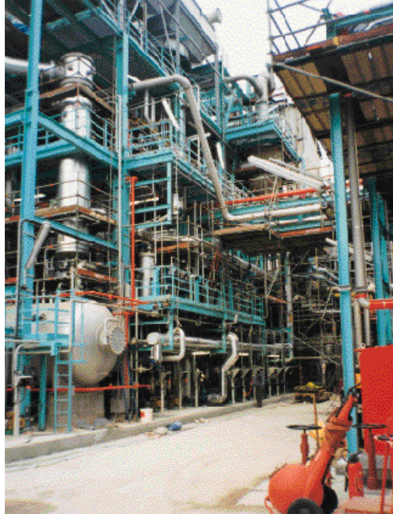
Port Jérôme rubber drying unit - France.
