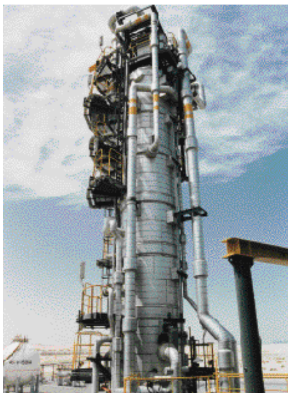
Fractionation column - OGD 1 - Abu Dhabi.
