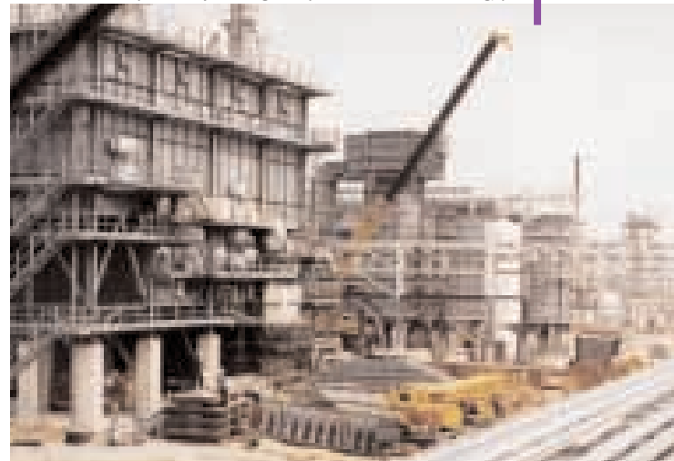
Naphtha reforming complex at Alexandria (Egypt).
