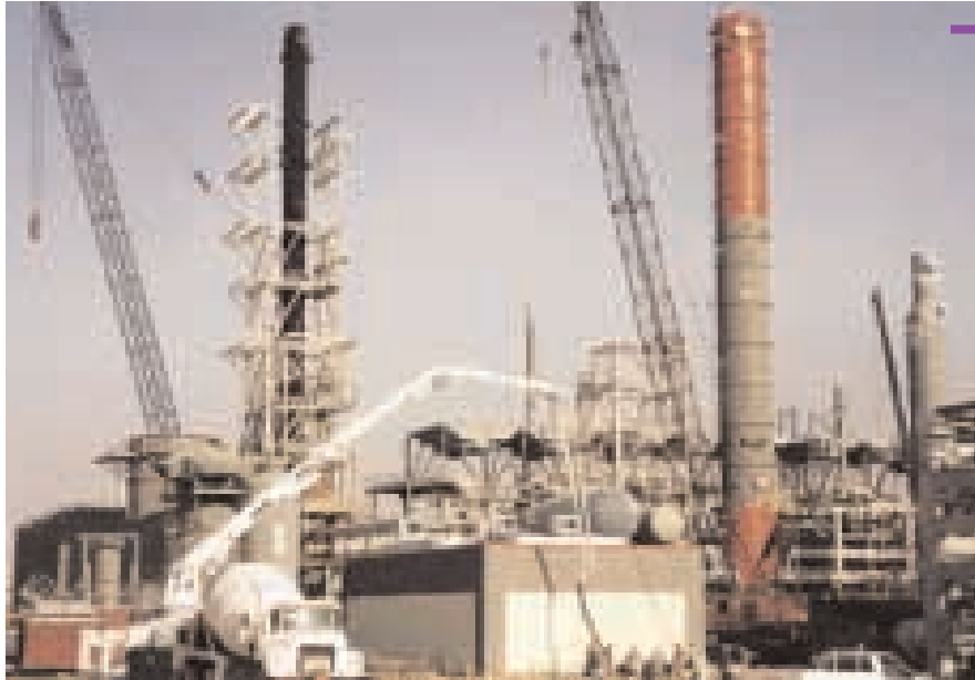
Isomerization unit and catalytic cracker at the MIDOR refinery (Egypt).
