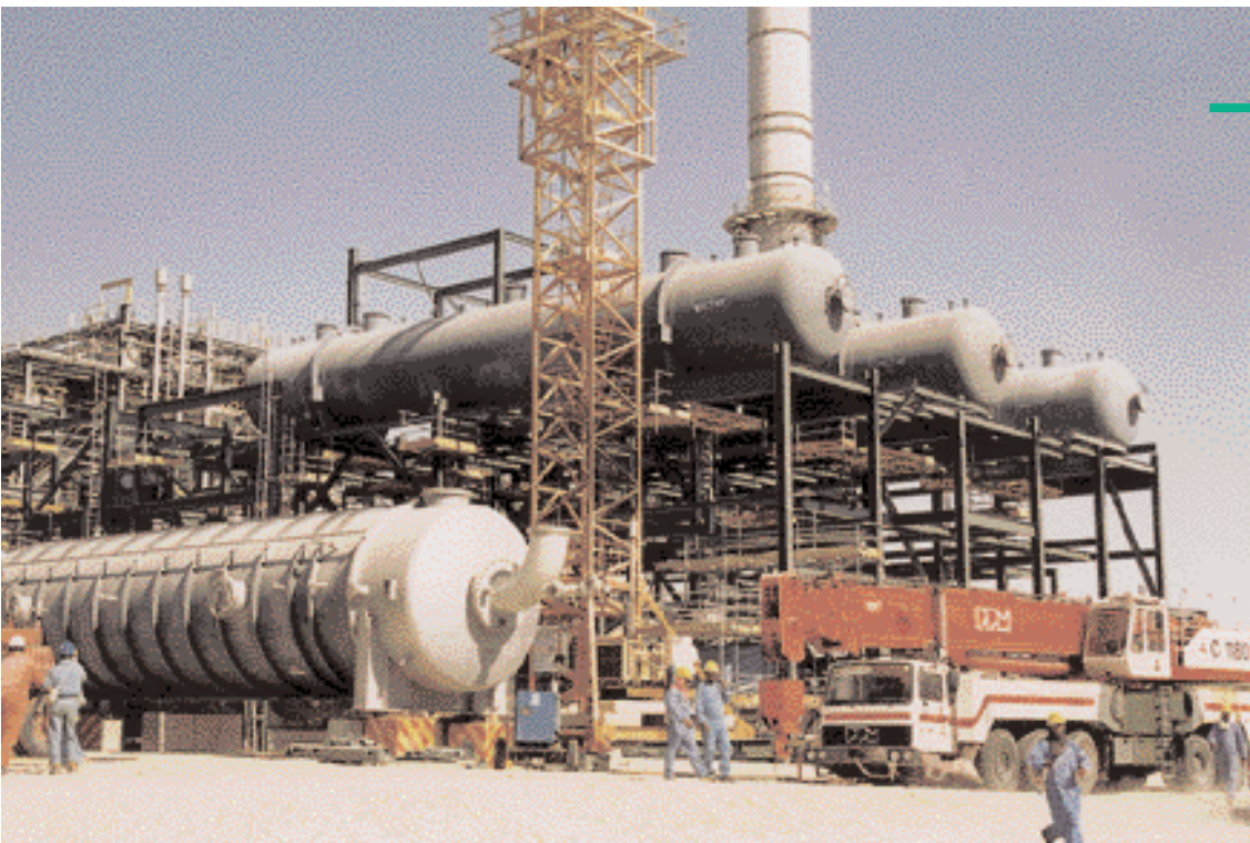
Sulfur unit at the "OGD 2" gas complex at Habshan (Abu Dhabi).
