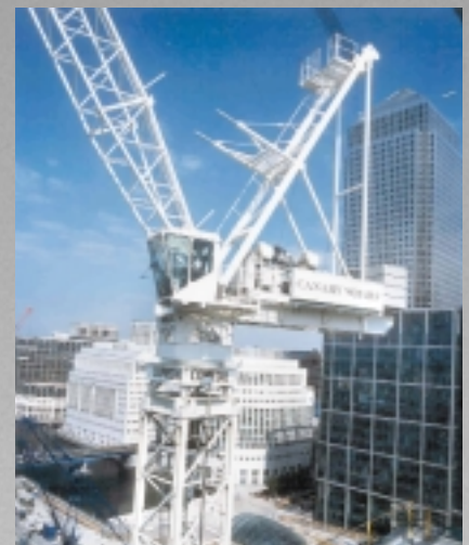
Right: The CC2800 Crawler Crane, a 600 metric ton crane manufactured by Demag being used by ENERCON, one of the largest windmill manufacturers in Germany.
