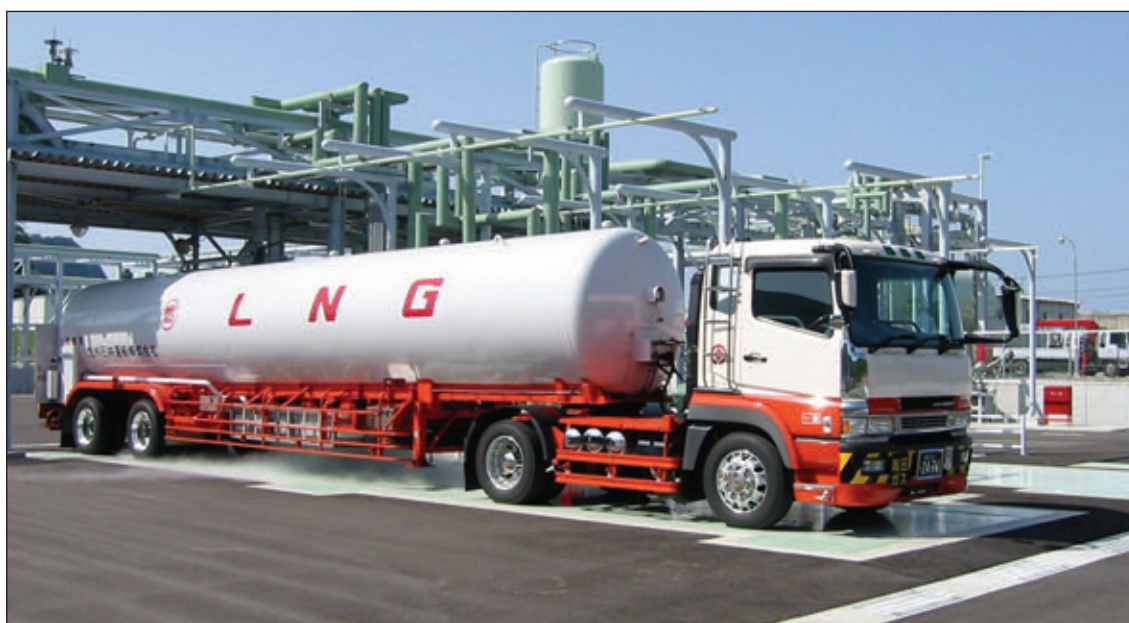
Road tanker loading facilities at the Nagasaki LNG terminal in Japan for supply of LNG to satellite storage installations.
