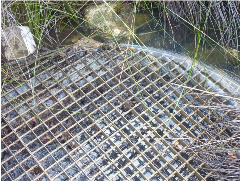
Figure 7. Water flowing from the wetland (W1) back into the drainage network via the bubble-up drain (taken 12/7/10).
