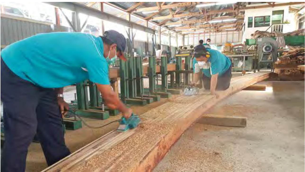
Meraut permukaan rasuk bagi membuat kemas dan rawatan Routing the surface of the beam to prepare for finishing and treatments
