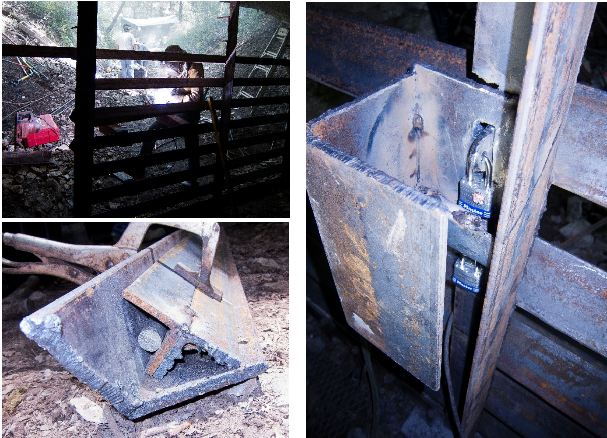
Figure 2. R.C. Schroeder welds one of the reinforced horizontal beams (top left). A pair of enhanced stiffeners inside the large angle iron (bottom left). The backside of the lock box with the dummy lock on the bottom and true lock on the top (right).
