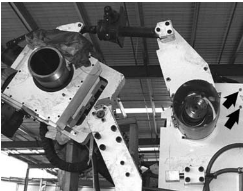
Figure 2.44 Airknife support head and its various adjustments. The arrows show where the flange bolts sheared off
