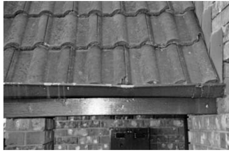
Figure 6.27 Photo showing the gutter and the locations on the gutter edge where some rubbing and deformation had occurred
