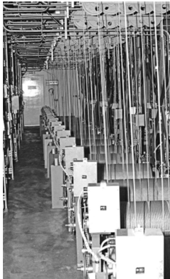
Figure 2.4 Winch floor showing the main winch drums and part of the pulley system
