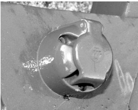
Figure 5.1 Typical trailer connector installed on a trailer
