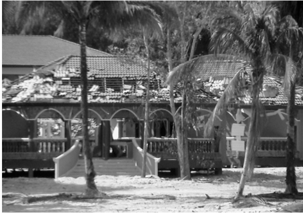
Figure 6 Damage up to a level of at least +9 m on roofs at Kamala Beach.
