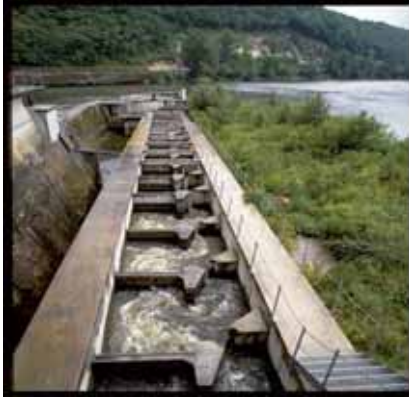
Photo 5. Vertical fish pass at Mauzac dam (left) and vertical fish passes at Iffezheim Dam (right) (Photo Larinier)
