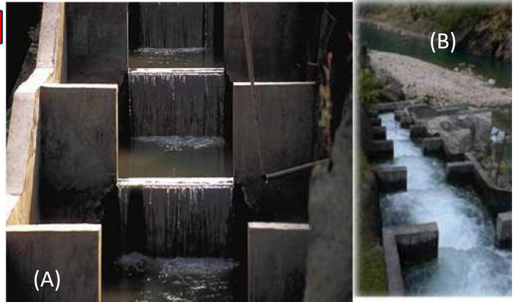
Fish ladder in (A) (Shrestha ) (B) Andhikhola
