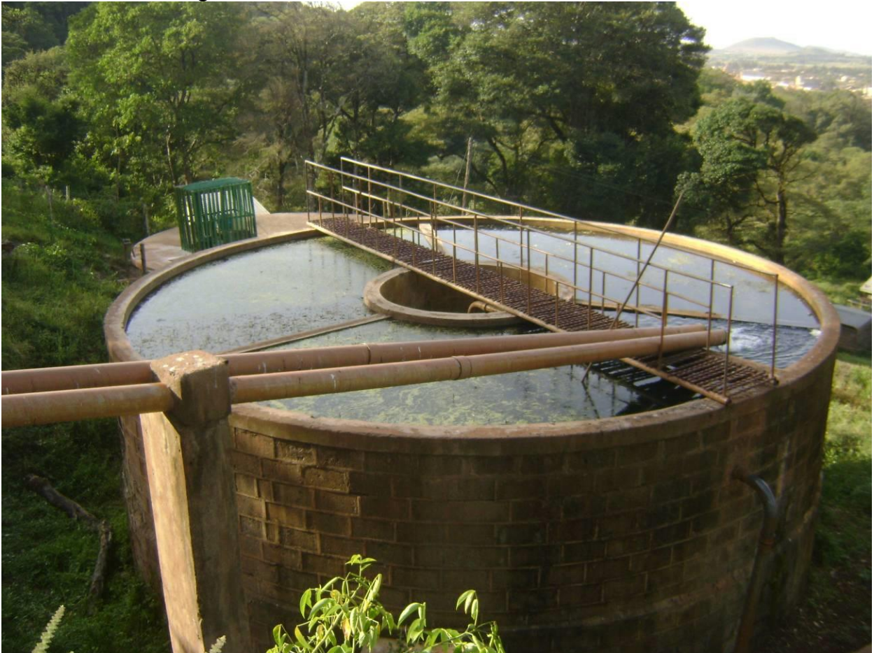
Plate 10:20-26m 3 /hr cfu with clear water tank hidden
