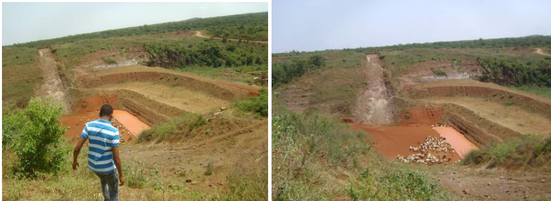
Plate 17: Stalled Badasa Dam
