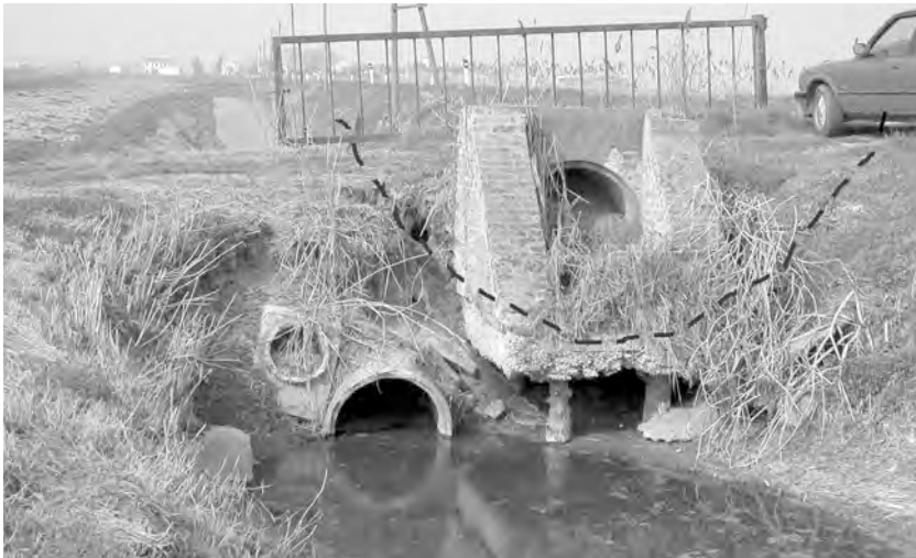
Fig. 5 – The effect of land subsidence in the Zennare Basin: an old masonry culvert presently above the water level and substituted by two lower concrete drainpipes, the higher of which already unusable. A qualitative position of the ditch section in the original configuration is sketched.
