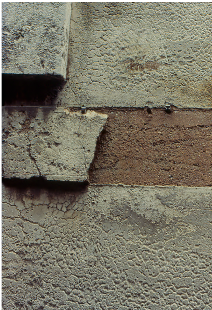
Fig. 5 - Venice, San Severo, Palazzo Cavagnis: marmorino applied on a preparation layer made of cocchiopesto (XVIIth century).
