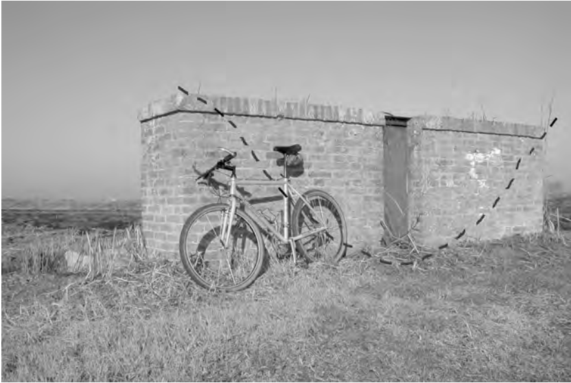
Fig. 4 – Effects of land subsidence in the Zennare Basin: an old abandoned weir originally constructed to close a drainage ditch completely protruded above the ground level. A qualitative position of the ditch section in the original configuration is sketched.
