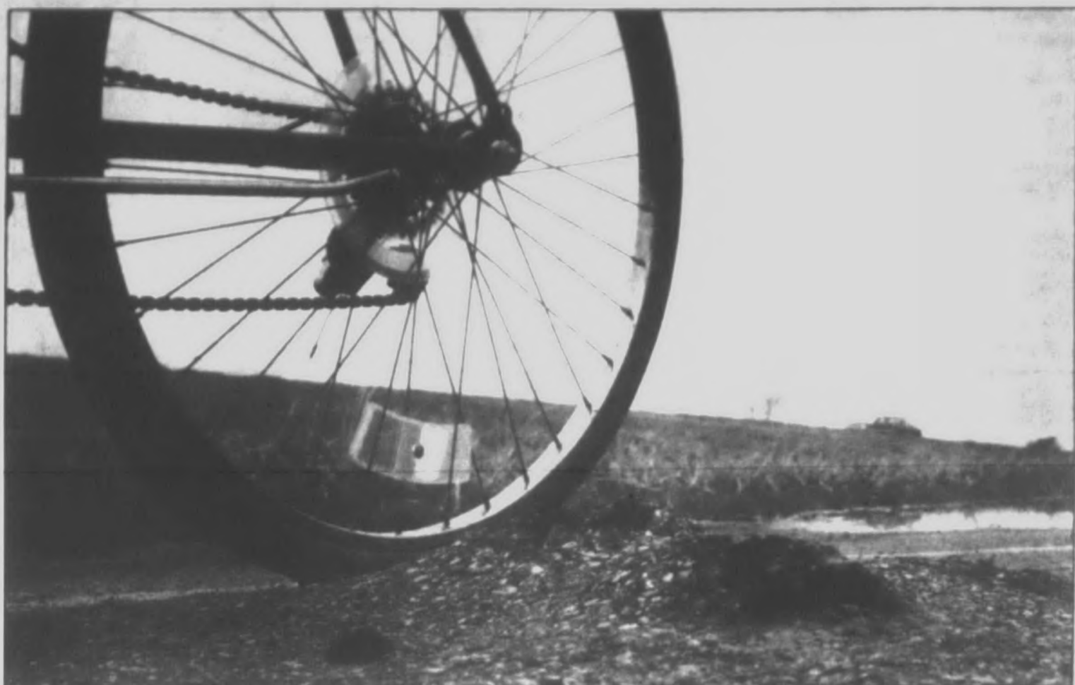
The asphalt and cement bike path along the I-275 expressway is showing its age. The longest recreational facility in the state was built in the mid-70s.
