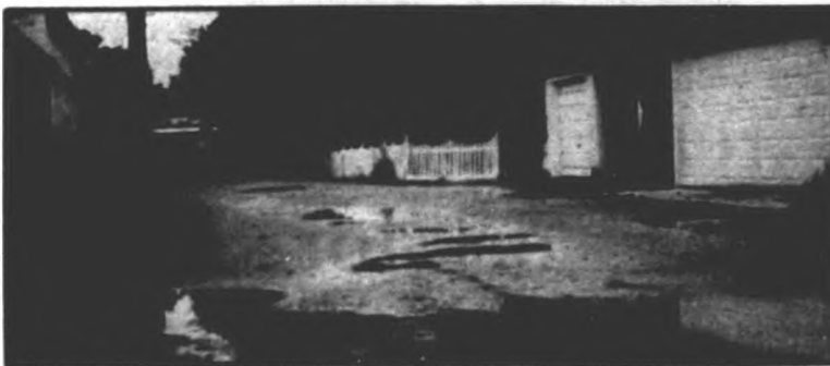
Water problem: Residents who share an alley near Sheldon Road are asking city commissioners to fix problems with the alley grade and a clogged storm drain.
