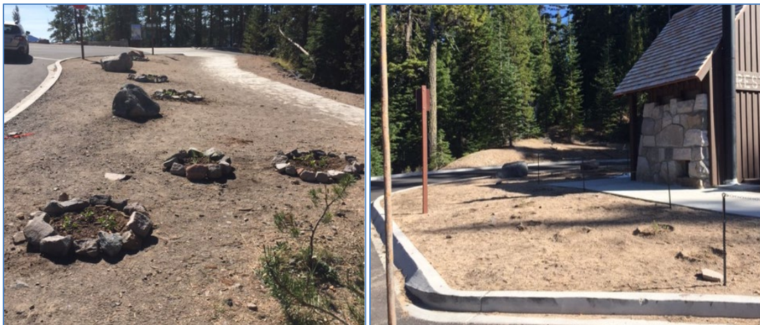
Figure 15. Plantings in groups with rock borders to mitigate trampling in heavily trafficked Cleetwood Cove parking lot areas (left). The area at the back of the Cleetwood Cove parking lot will be adjusted to allow for RVs to drive around the comfort station (right). Photos by Carrie Wyler.
