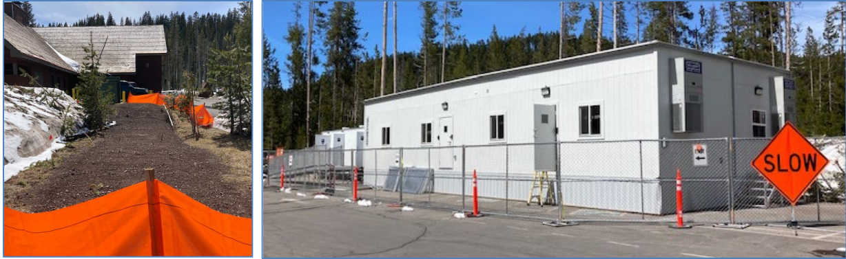
Figure 4. Ground disturbance near the Temporary VC where underground cables and piping were installed (left). Temporary VC and restrooms located at Mazama Village (right). Photos by Carrie Wyler.
