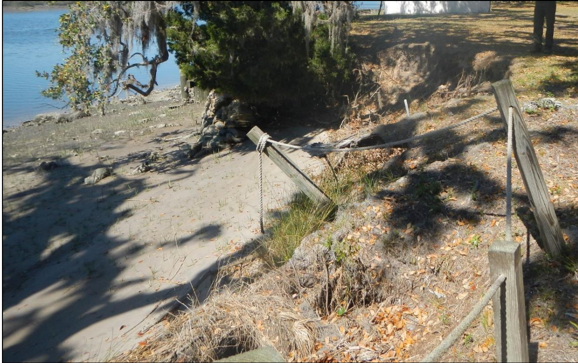
Figure 15. “End-around” erosion south of a stabilized shoreline area at Plum Orchard (SMUMN GSS photo).
