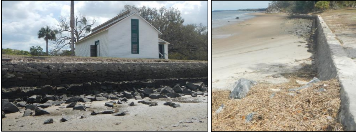
Figure 96. The Dungeness seawall at low tide (SMUMN GSS photo).
