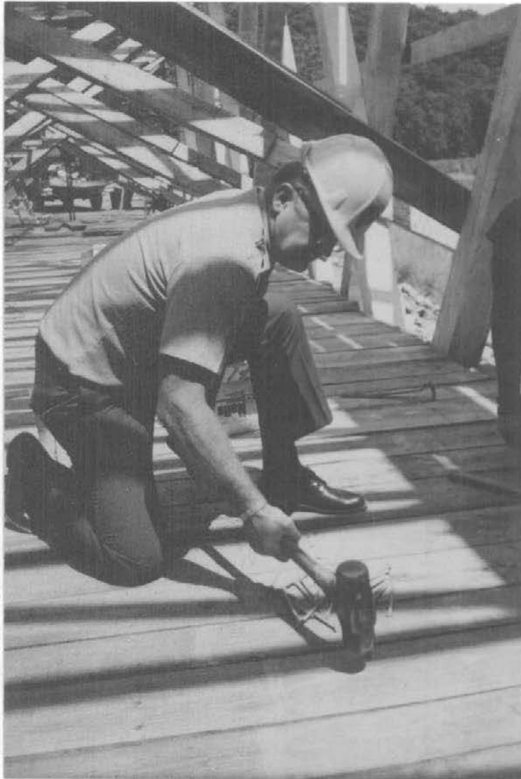
Figure 41: Assistant Superintendent, Operations, Einar L. Johnson drives a nail into the reconstructed Everett Road Covered Bridge, a project undertaken by the National Park Service's Williamsport Preservation Training Center.
