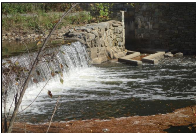
Rock Creek, showing fish ladder for shad and herring (ROCR). Photo credit: S.J. Fiske
