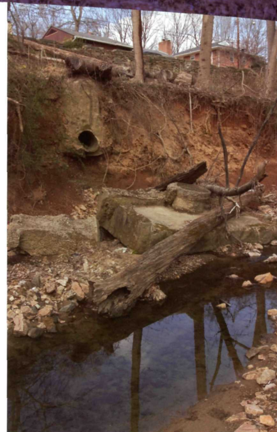
Figure 3 Storm water flowing into an unprotected gully causes massive erosion.
