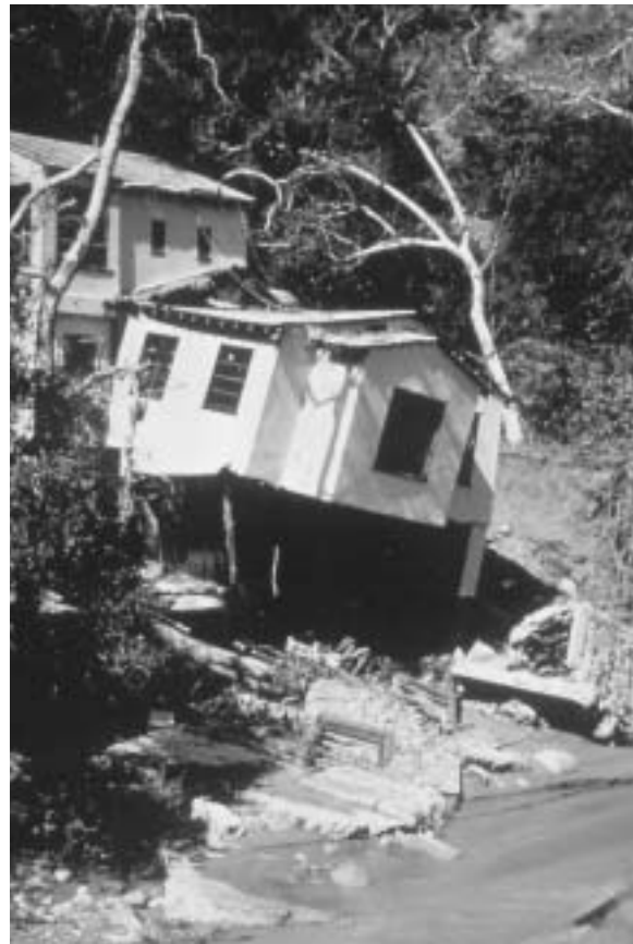
Slope failure in Topanga Canyon (NPS photo).
