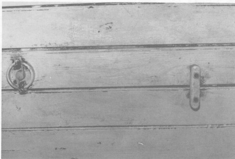
FIGURE 34. Knob and tube wiring system remnants.
