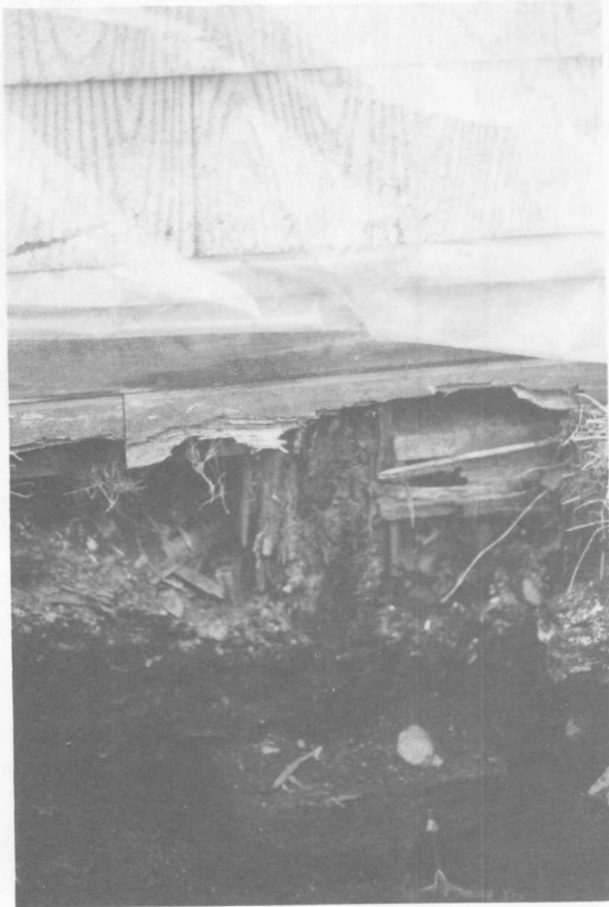
FIGURE 29. Rotted timber pier at south wall.
