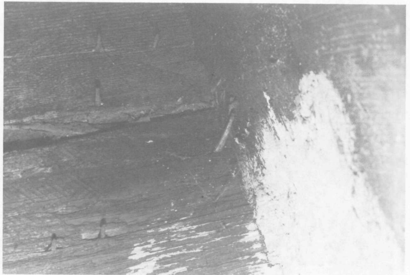
FIGURE 33. Cut nails used to secure spaced sheathing to rafters. Wire nails used to attach shingles to sheathing.
