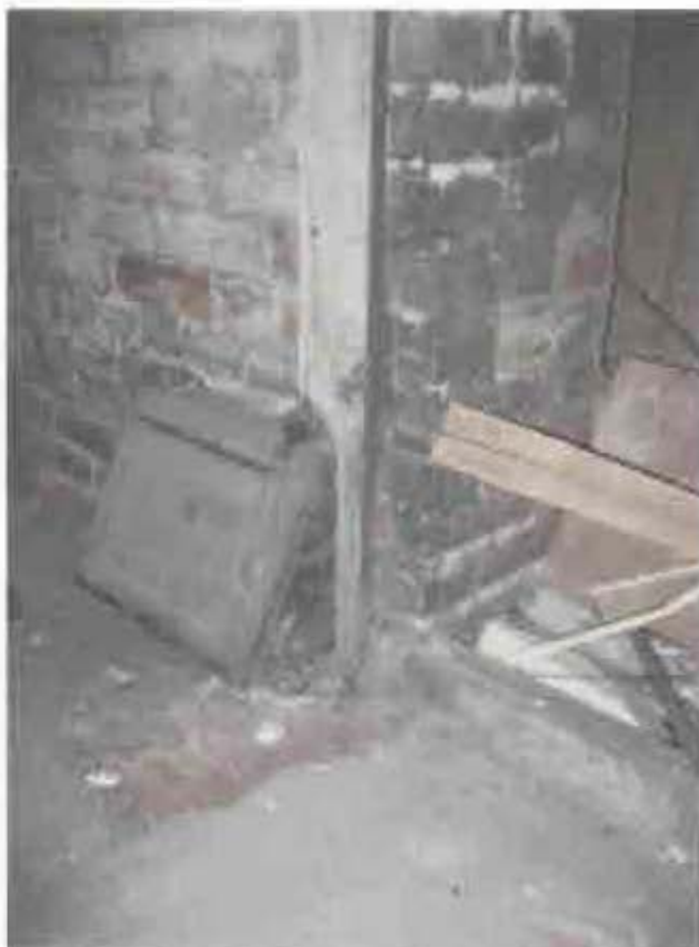
Figure 2.16. Room 001, view of brick flooring, and cast-iron door on east side of room 001a (central brick furnace chamber).
