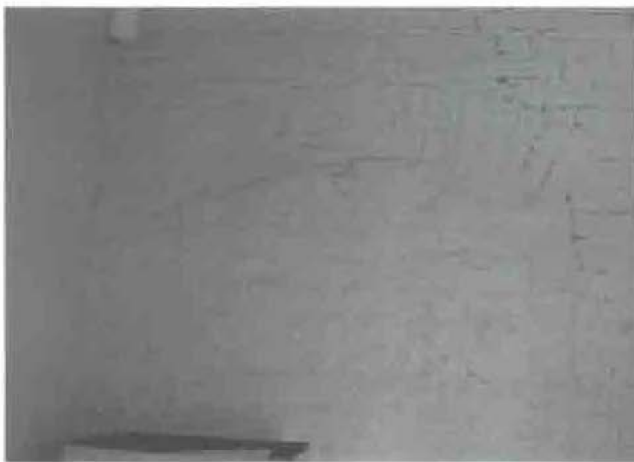
Figure 2.50. Room 115 in the 1938 addition, north wall, infilled arched window opening in brick wall of former carriage house.
