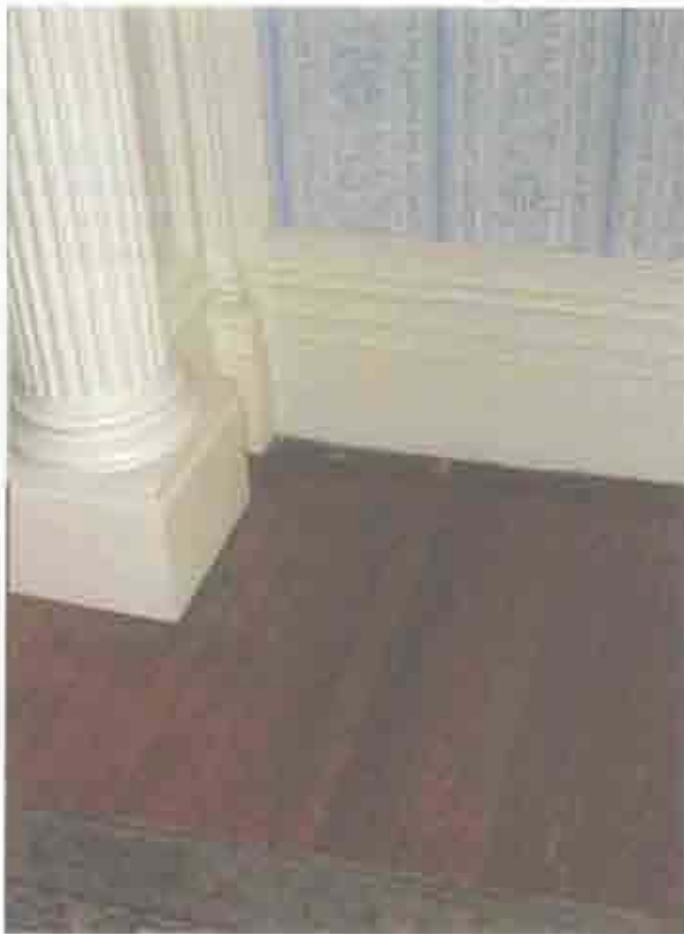
Figure 2.44. Room 108 (Dining Room), unidentified floor feature.
