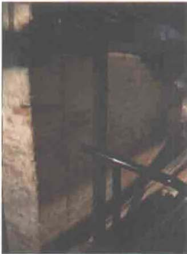
Figure 2.23. Room 001, view of unstable west wall of room 001a (central brick furnace chamber).
