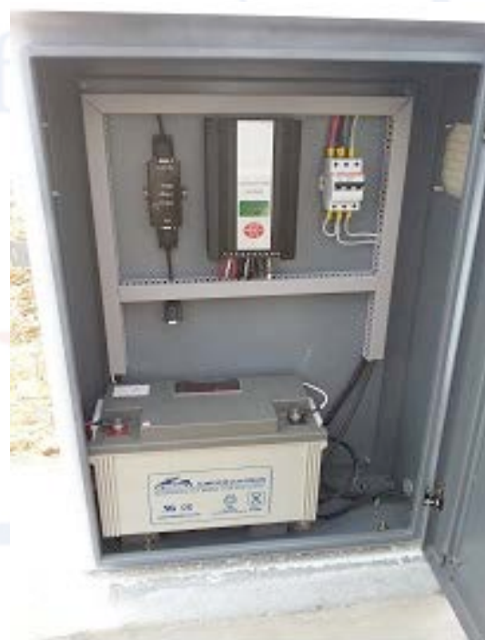
b) Equipment within the cabinet
