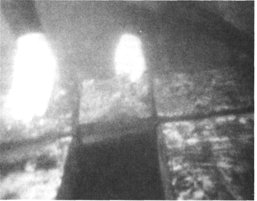
16 Ceiling planking cut between frames to permit access to the exterior planking.
