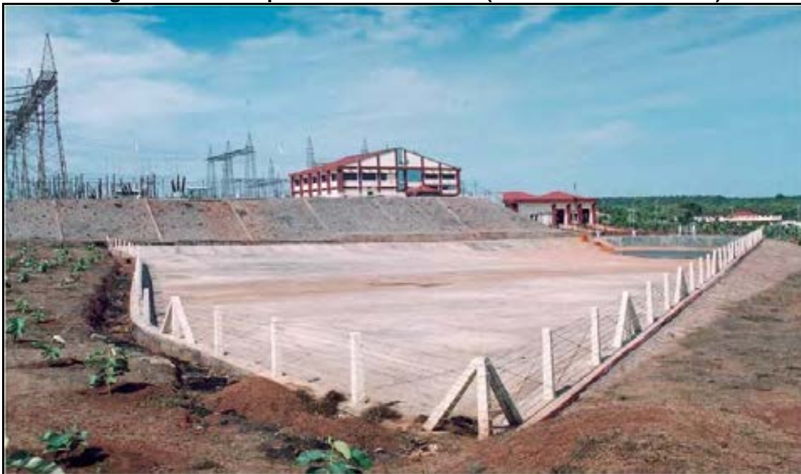
Figure 6.14: Example of Retention Pond (at electrical substation)
