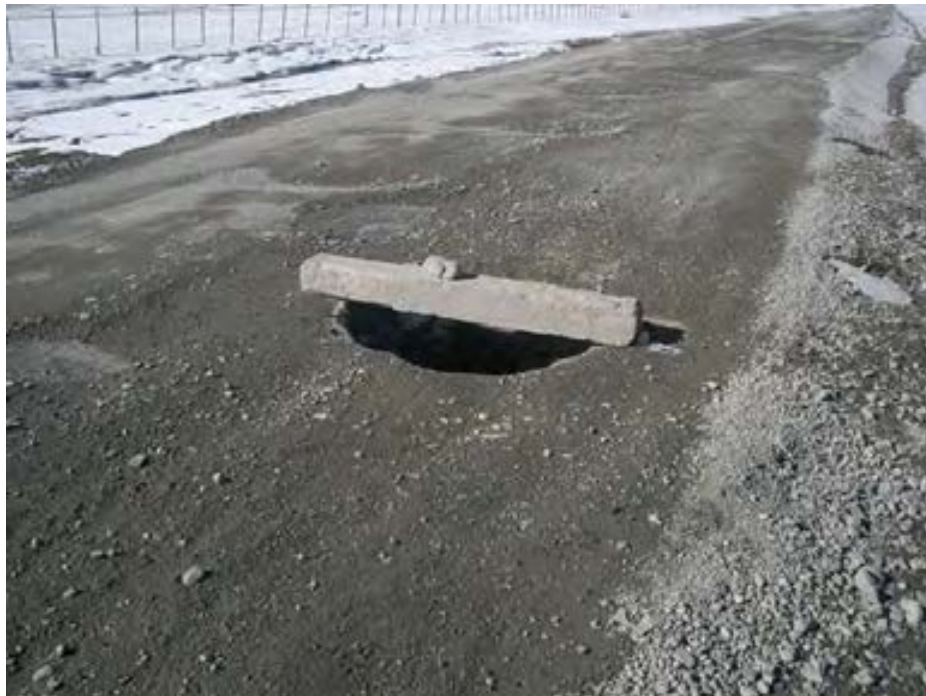
Hole on the box culvert (16 October 2009)
