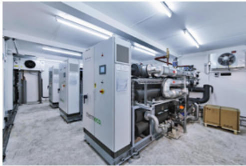
Heat pump in the abattoir of Zurich
