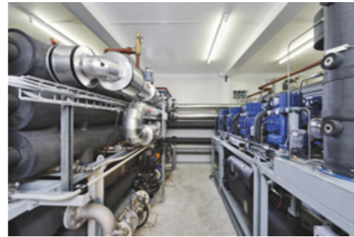
Heat pumps with GEA Bock CO 2 compressors
