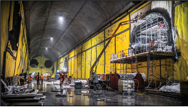
$1.0B East Side Access CM006 & CM007 Projects ▲ Metropolitan Transportation Authority New York, NY
