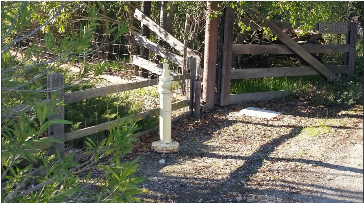
Existing fire hydrant
