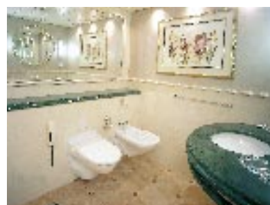
Several cruisers also use Evac vacuum systems. In the photo the Royal suite restroom in the M/S Grandeur of the Seas.
