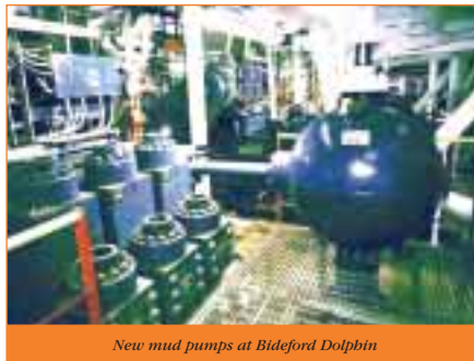
New mud pumps at Bideford Dolphin
