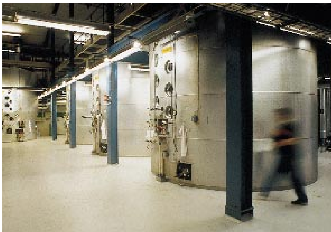
The sugar boiling station at Arlöv Sugar Refinery.
