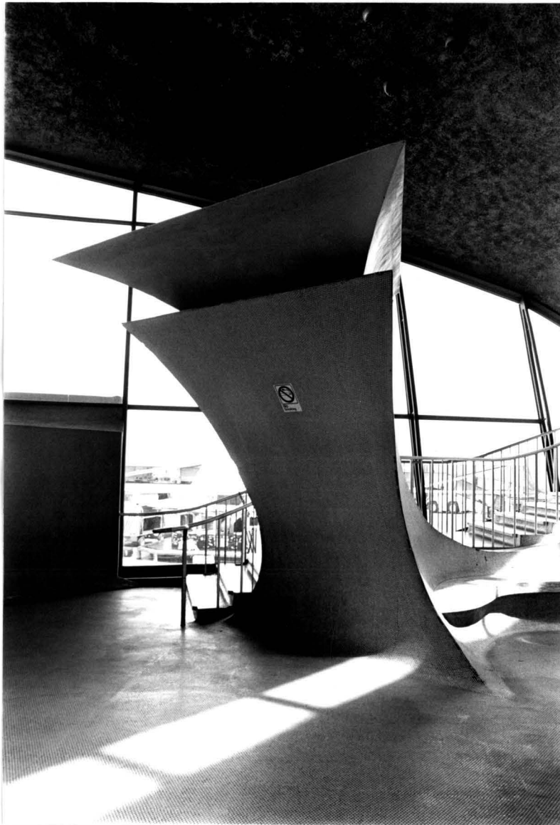
"Air Fountain" ventilation duct. Trans World Airlines Flight Center at New York International Airport Interior. TWA Flight Center Interior, John F. Kennedy International Airport, Queens.
