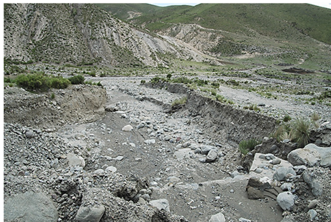
Photo 12: Road collapsed between Amaicha del Valle and Tafi del Valle.
